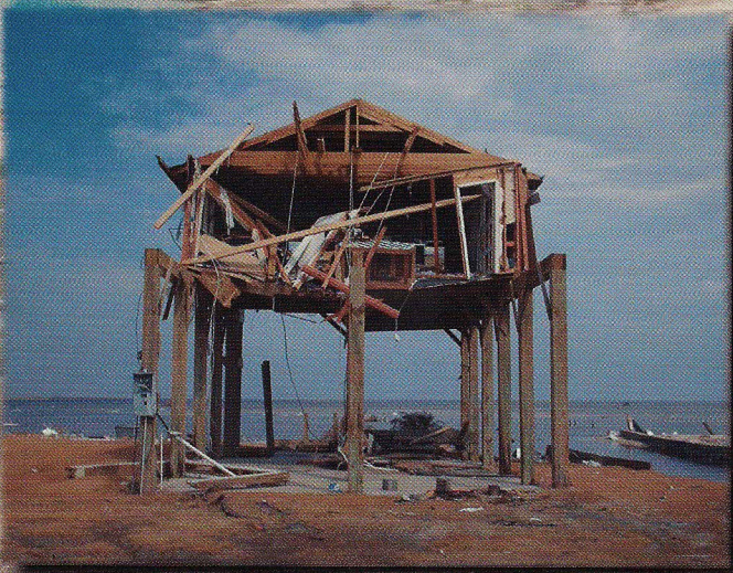
Home destroyed by storm surge from Hurricane Ike near Caplen, TX.
